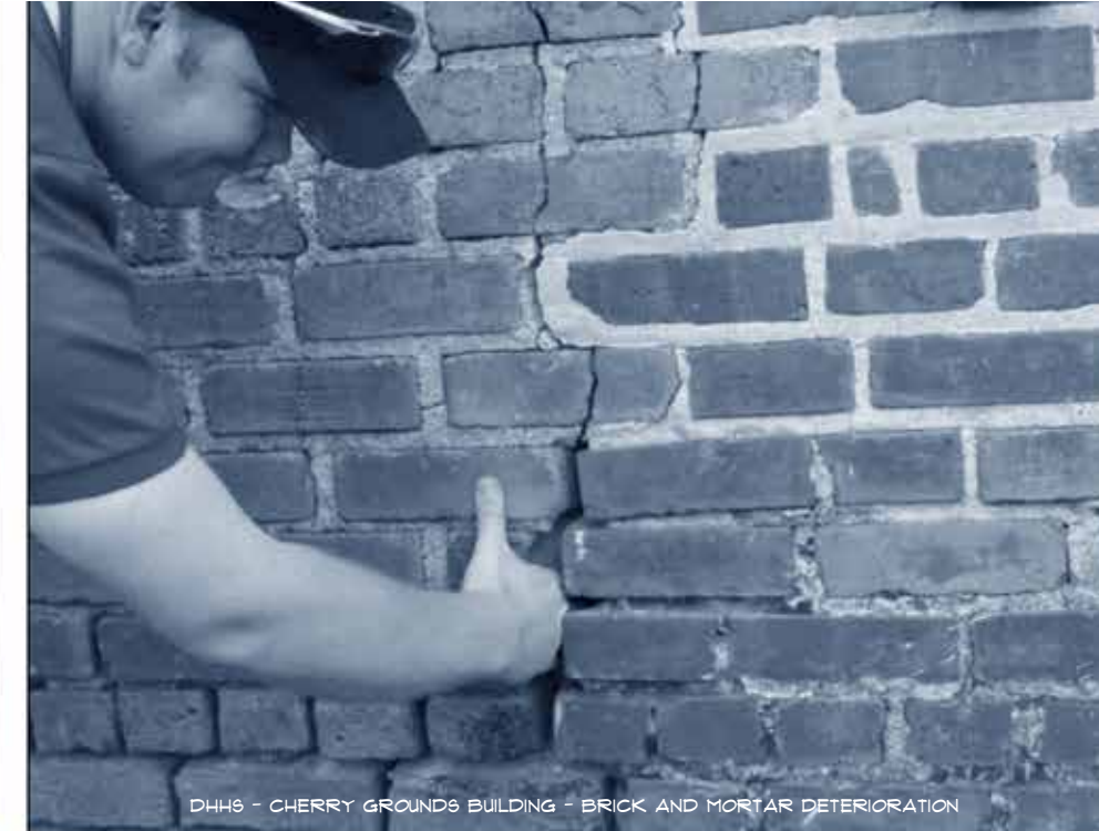
DHS - CHERRY GROUNDS BUILDING - BRICK AND MORTAR DETERIORATION
