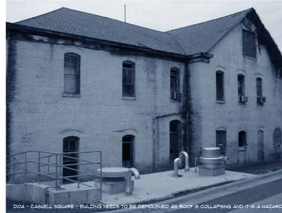
DOA - CASWELL SQUARE - BUILDING NEEDS TO BE DEMOLISHED AS ROOF IS COLLAPSING AND IT IS A HAZARD
