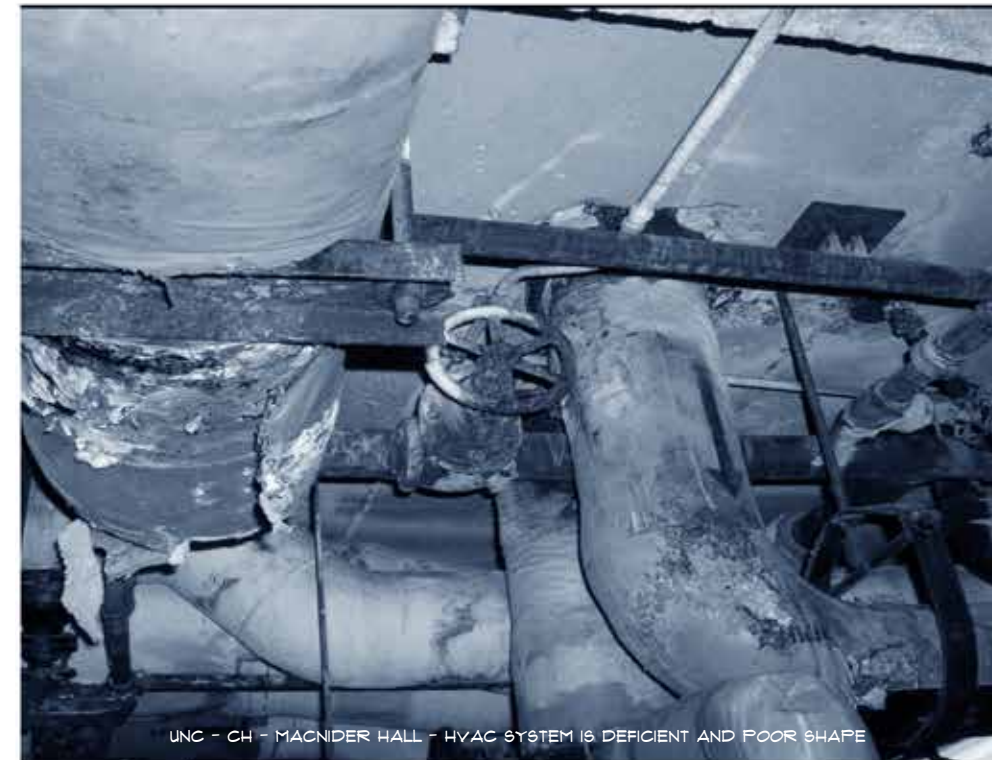
UNC - CH - MACNDER HALL - HVAC SYSTEM IS DEFICIENT AND POOR SHAPE
